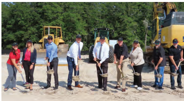
BARRETTE breaks ground on its Brooksville, FL., recycling plant that will bring nearly 170 new jobs to the region.
